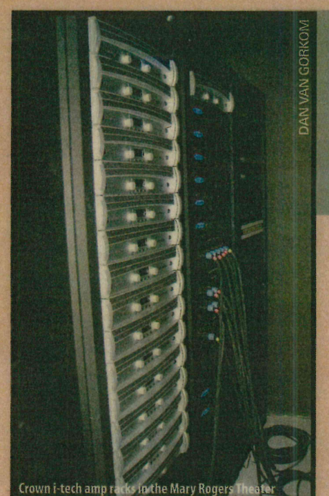
Crown i-tech amp racks in the Mary Rogers Theater
